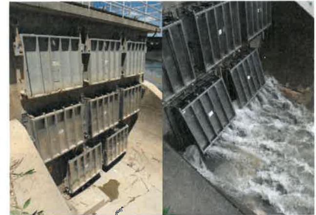
CSO #005 in South Fairmount under dry and wet weather conditions.
